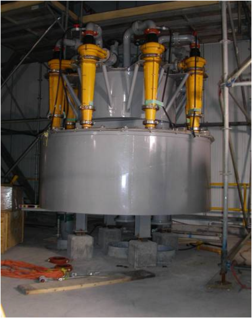
Primary Hydroclone Bank
