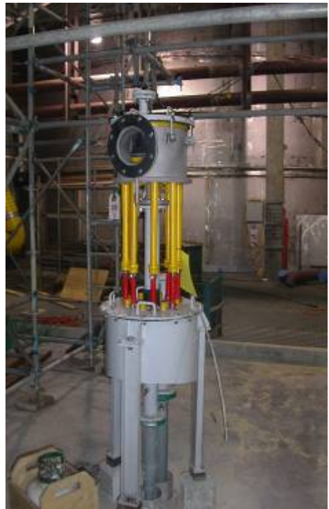
Secondary (Purge) Hydroclone Bank
